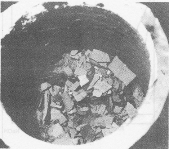
Fig. 8. Scaling of superheater tube.
