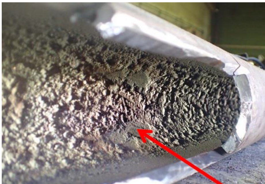
Figure 34. Internal deposits inside a boiler tube (internal report form Isberg, 2018).
