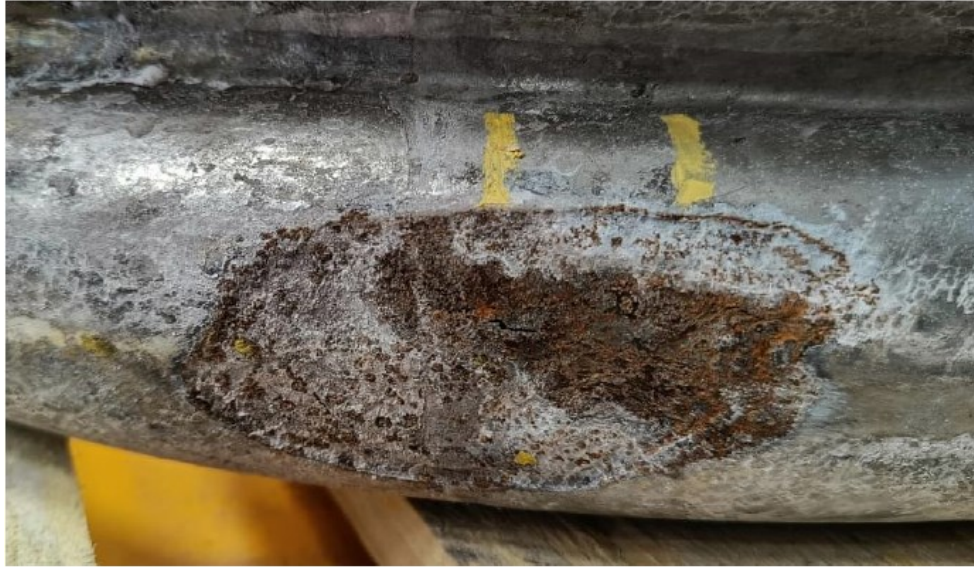
Figure 30. Corroded and ruptured wall tube due pitting corrosion and pressure (internal report from Inkinen et al., 2024).
