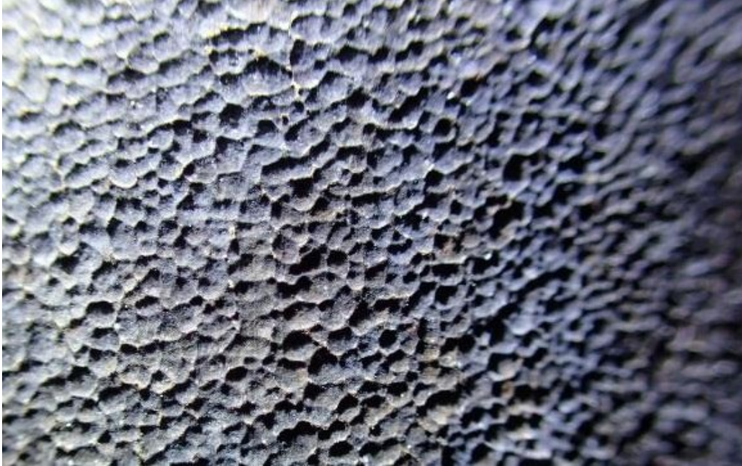
Figure 28. Corroded stainless steel cladding (internal report from Isberg, 2018).
